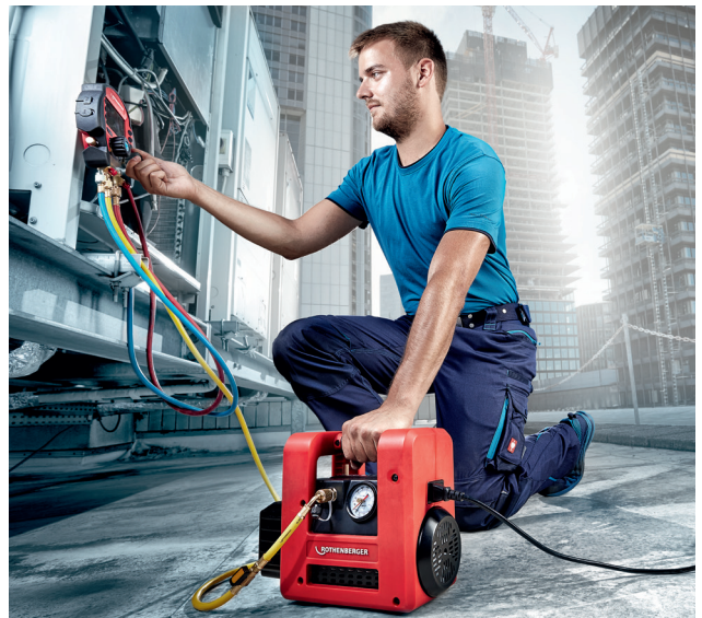
ROAIRVAC R32 1.5 - vacuum pump in use with the digital manifold ROCOOL 600
